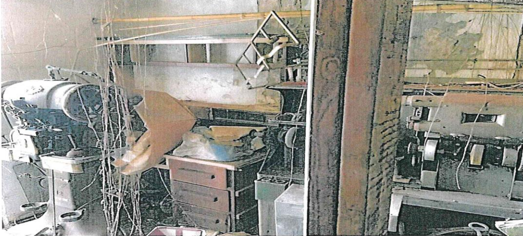
File Name: IMG_1334 Violation Code: 311.3 Specific Location: Throughout building Inspected Date: 2023-09-08 12:44:21
