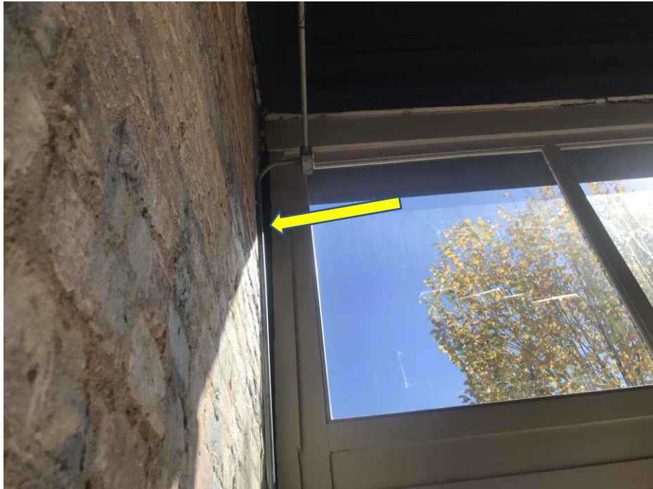
Photo 1: Gap that is approximately 2-1/2" wide has formed at the ceiling level of the building's front right corner (as seen from the neighboring building, 315 W. Main St.)
