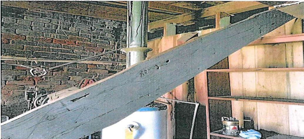
File Name: IMG_1333 Violation Code: 311.3 Specific Location: Throughout building Inspected Date: 2023-09-08 12:44:21
