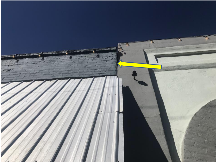
Photo 3: Building's front side brick parapet is significantly leaning outward
