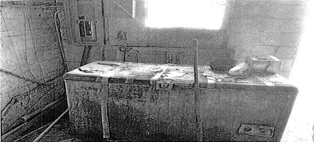
File Name: IMG_1336 Violation Code: 311.3 Specific Location: Throughout building Inspected Date: 2023-09-08 12:44:21
