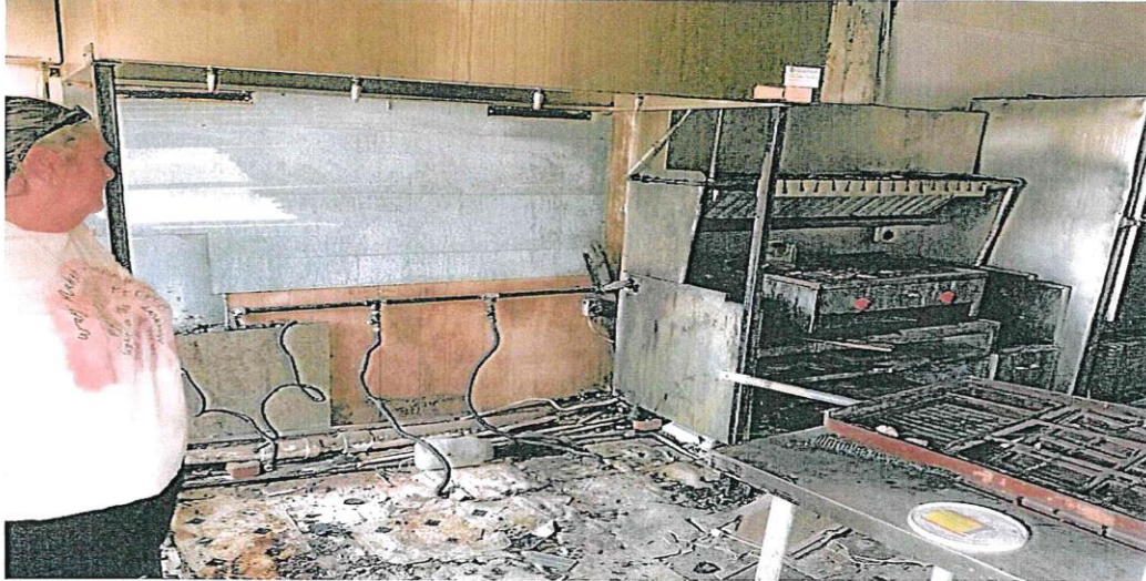
File Name: IMG_1310 Violation Code: 311.3 Specific Location: Throughout building Inspected Date: 2023-09-08 12:44:21
