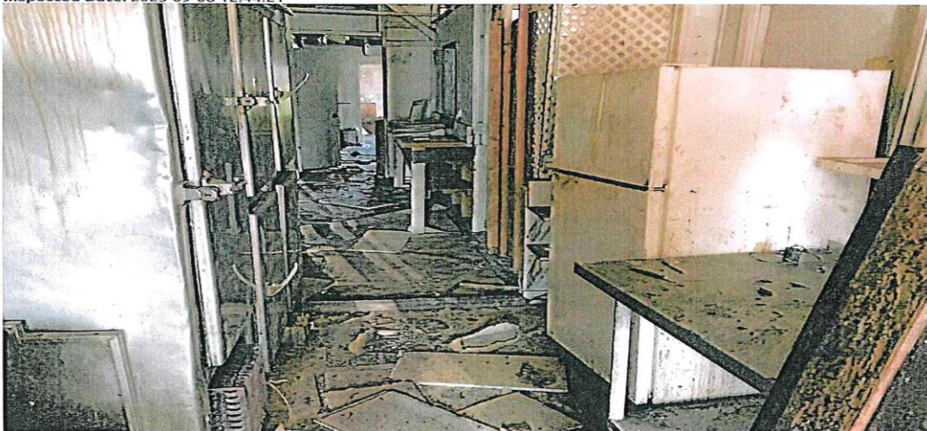
File Name: IMG_1321 Violation Code: 311.3 Specific Location: Throughout building Inspected Date: 2023-09-08 12:44:21
