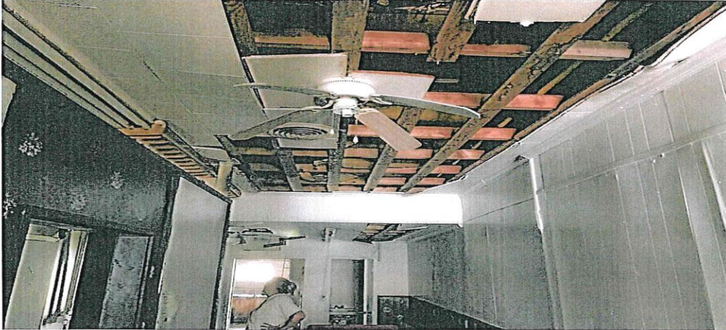
File Name: IMG_1327 Violation Code: 311.3 Specific Location: Throughout building Inspected Date: 2023-09-08 12:44:21
