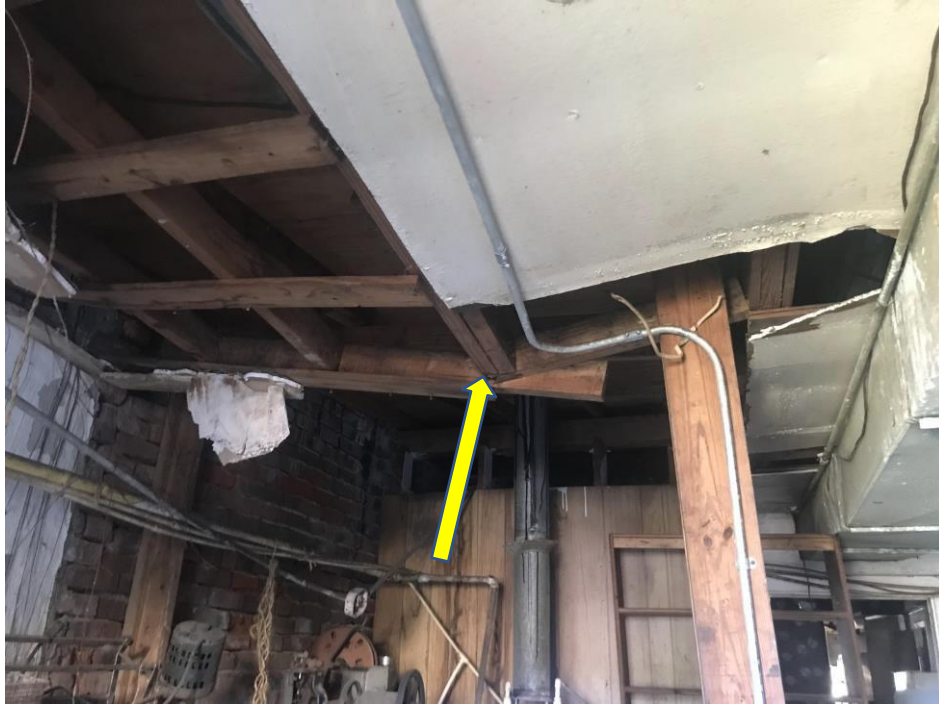
Photo 5: Collapsed roof structure near the building's rear side wall
