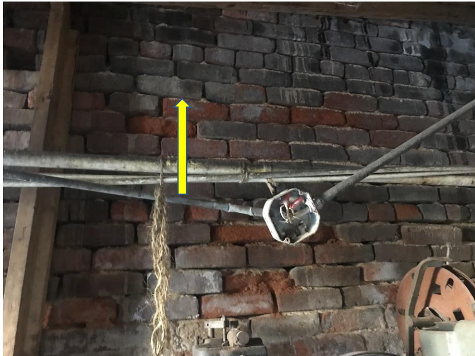
Photo 6: Significantly deteriorated mortar along the building's right side masonry wall, typical
