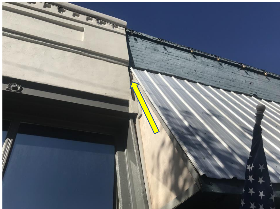
Photo 2: Gap that is approximately 2-1/2" wide has formed at the ceiling level of the building's front left corner, exposing a potential wooden beam that supports the front side brick parapet
