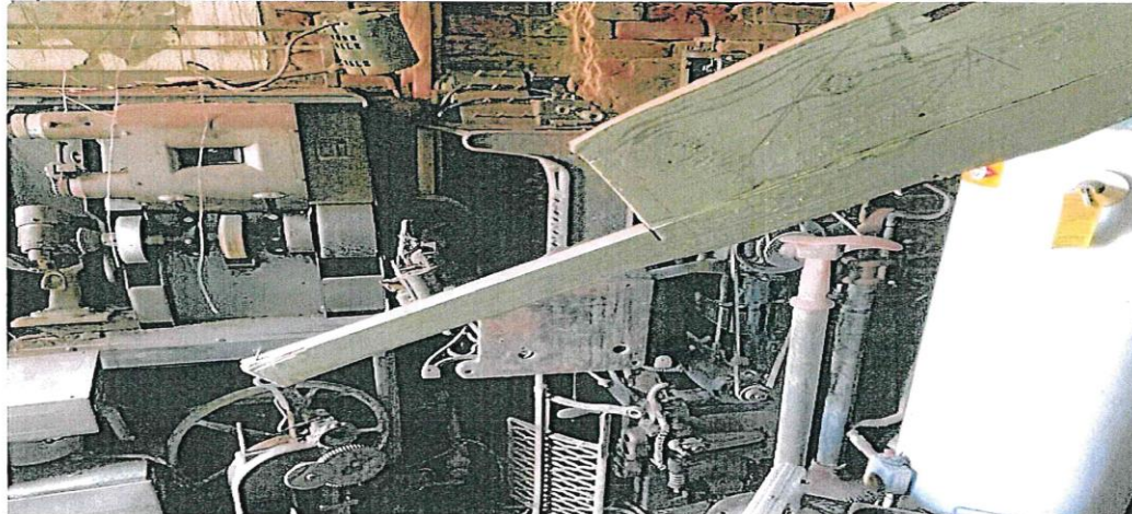
File Name: IMG_1335 Violation Code: 311.3 Specific Location: Throughout building Inspected Date: 2023-09-08 12:44:21
