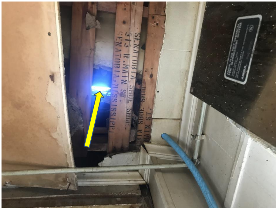
Photo 4: Outward leaning brick parapet has caused a gap to form between the noted parapet and the roof structure along the building's front side wall
